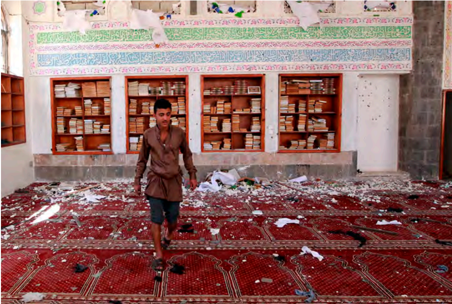
Figure 13.9 A Yemeni man inspects the damage following a bomb explosion at the Badr mosque in southern Sana'a on 20 March 2015. Image: Mohammed Huwais / Getty Images
